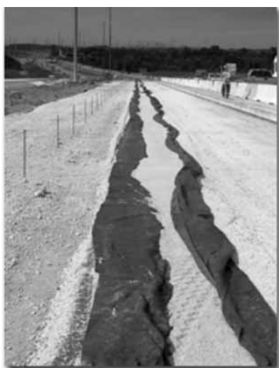
Figure 2.11: Non-woven geotextiles is being used in a drainage application during roadway construction
