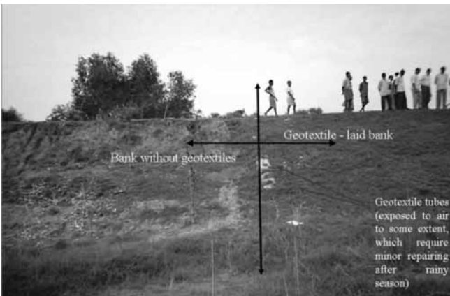
Figure 3.1b: Condition of river bank with and without geotextiles
